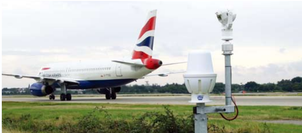
▲ Radar technology, along with integrated surveillance and security systems, helps ensure 24/7 security at airports under all weather conditions. (Image courtesy of Navtech Radar)
